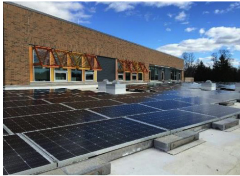
Solar Array at Discovery Elementary School
